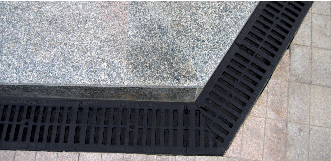
On the city streets, drainage gutters BGU with cast-iron grates
