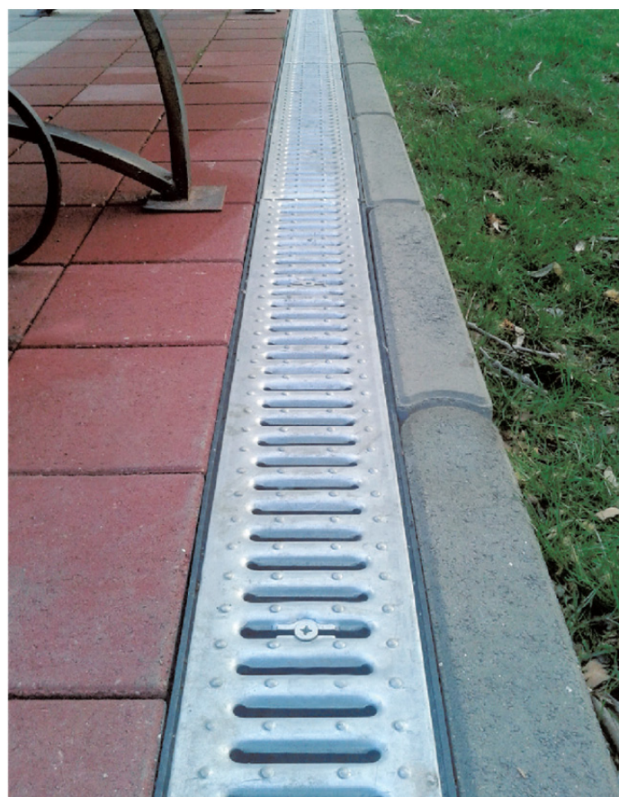
Urban park, drainage gutters Gidrolica® Standart with galvanized grates
