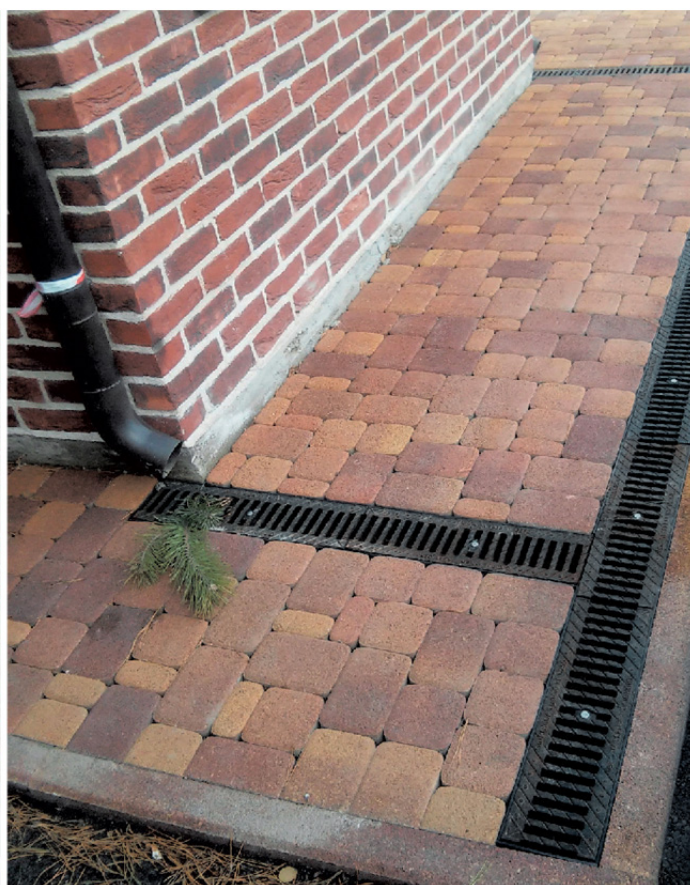
Detached house, drainage gutters Gidrolica® Standart with cast-iron grates
