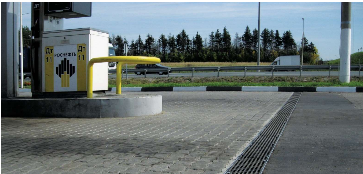
Rosneft, filling station chain, drainage gutters BGU-Z with cast-iron grates
